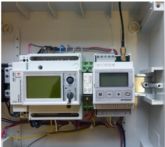
Figure 1 FLTA in fixed installation
